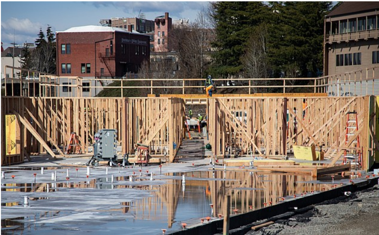
The Millworks project begins construction at the downtown waterfront. The building will have affordable housing and child care. (Hailey Hoffman/Cascadia Daily News)
