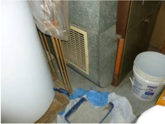
This is not a good location for a return air duct. If upgrading furnace move this to a cleaner location.
