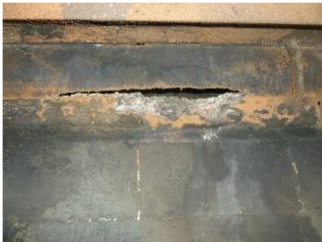
Significant corrosion on the fireplace damper.
