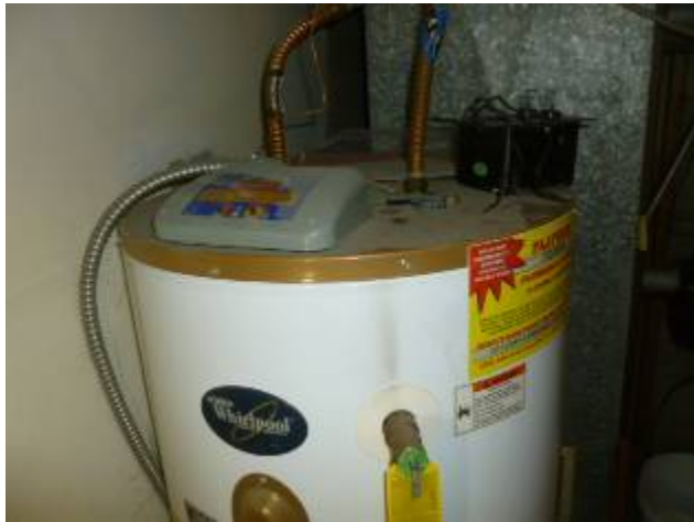
Standard electric water heater.
