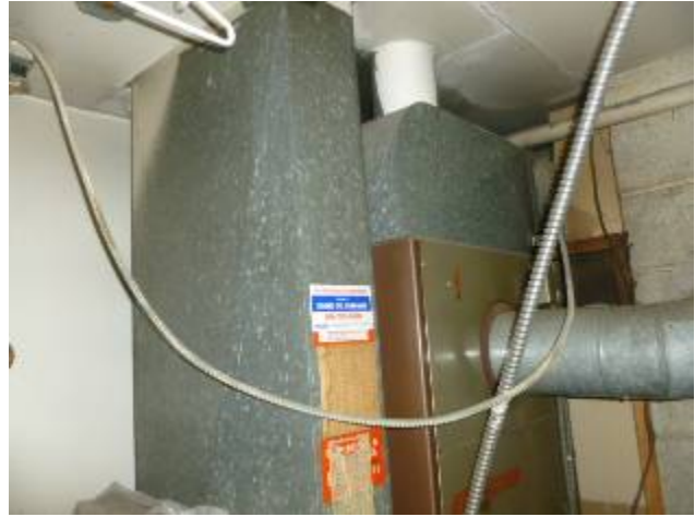
Metal ducts are inside conditioned space.
